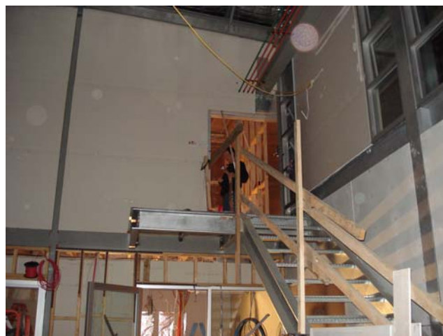
Figure 4. Measuring attenuation around the screened room door from the stair landing
