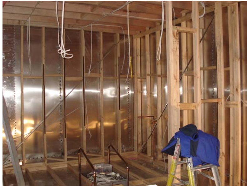
Figure 1. Inside the STI screened room during construction. Note the welded seams between the adjacent aluminium lining panels.
